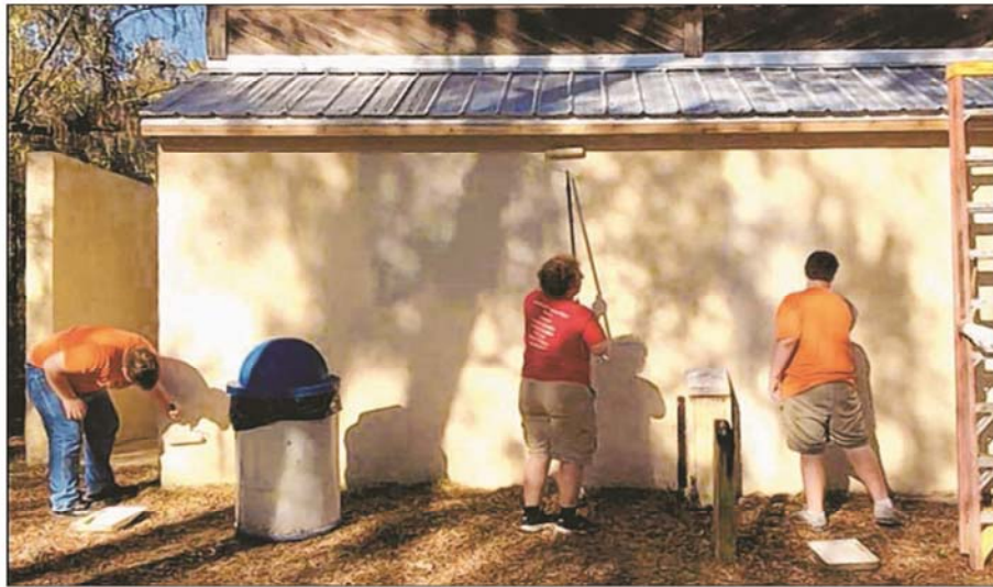
Members of Boy Scout Troop 457 paint the restroom building, after the new roof was installed. From left are Christian Mysilwiec, Ben VanDermark and Vito Delgorio. You can find more photos on page D5. Special to the Chronicle
